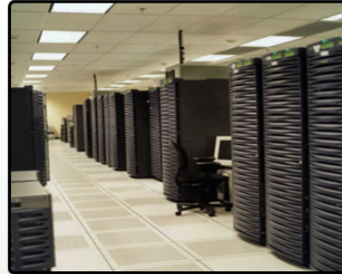
Hewlett Packard Cloud Computing Container
